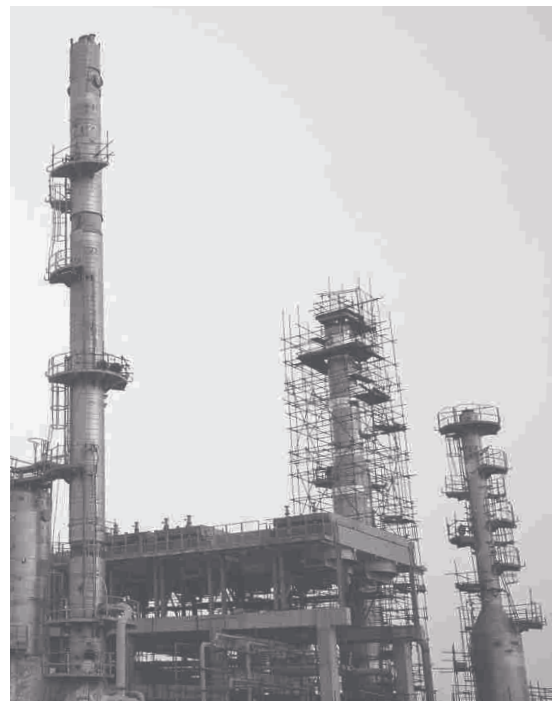
BOPL, an associated company of BPPL is reaching completion at a fast pace
