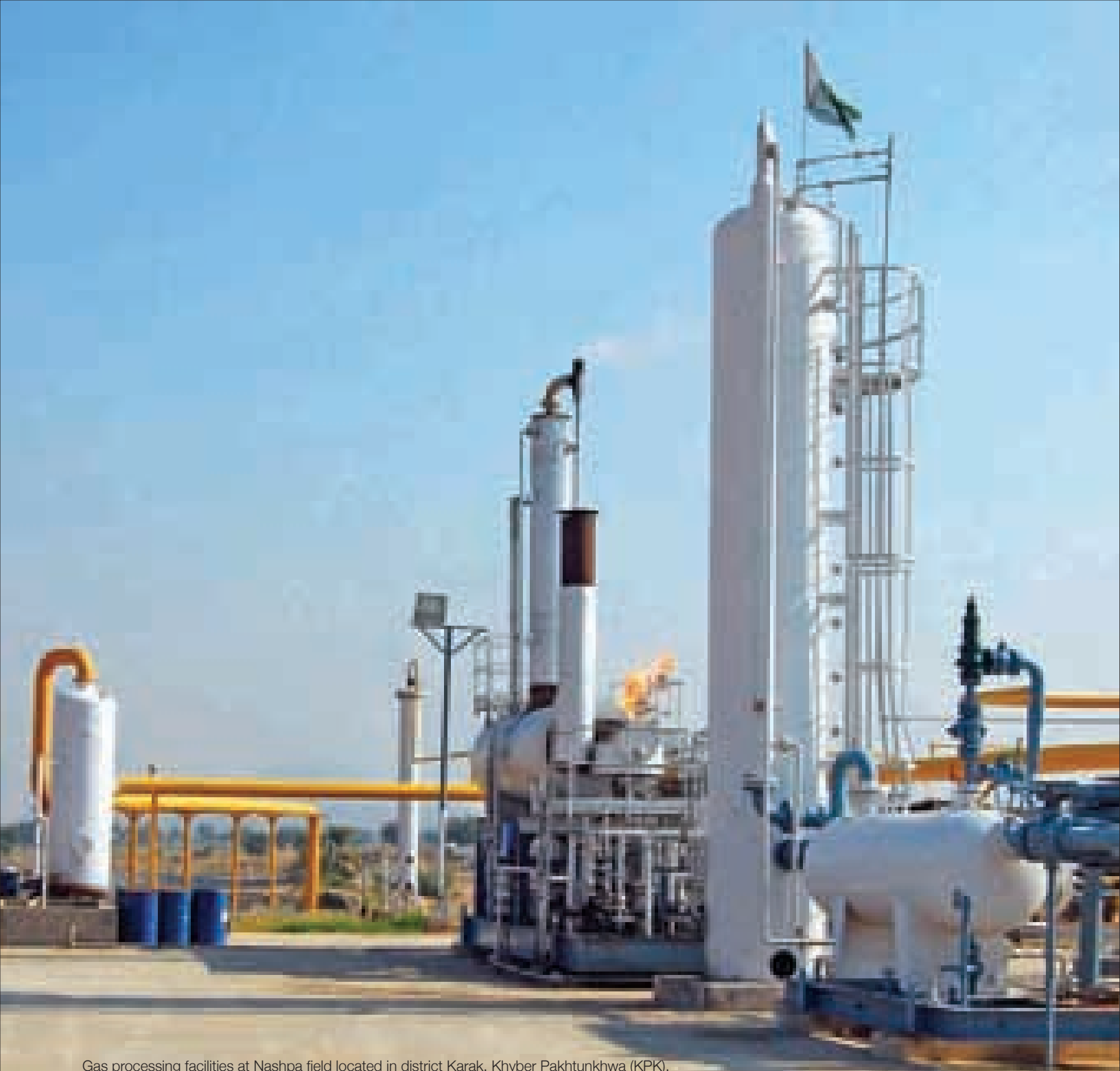
Gas processing facilities at Nashpa field located in district Karak, Khyber Pakhtunkhwa (KPK).
