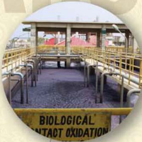
First ETP (Effluent Treatment Plant) in the textile sector
