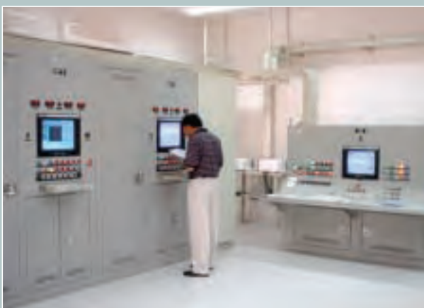
The new control room of the 17,000 HP compressors station relocated from Sui and Shikarpur to Hyderabad using latest digital control systems.
