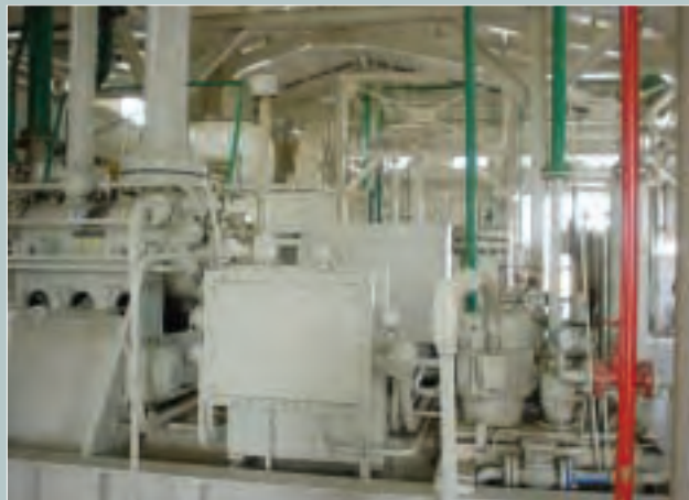
Sibi Compressor Station, vital for pumping additional gas to Balochistan.
