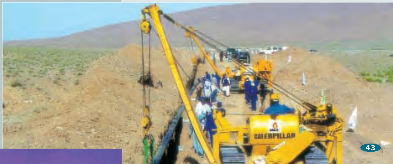
Work in progress on the Ziarat Gas Pipeline, laid in difficult mountainous terrain.
