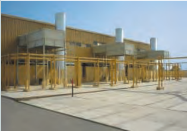
New Hyderabad Compressor Station ensuring increased quantities of Gas to meet the additional requirements of power & industrial sector.
