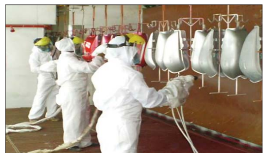
Electrostatic painting in new paint shop
