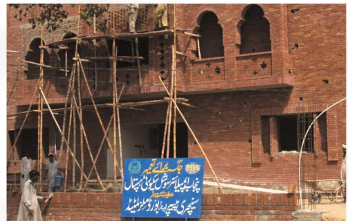
Mini - Hospital construction in progress on land donated by Century Paper & Board Mills Limited
