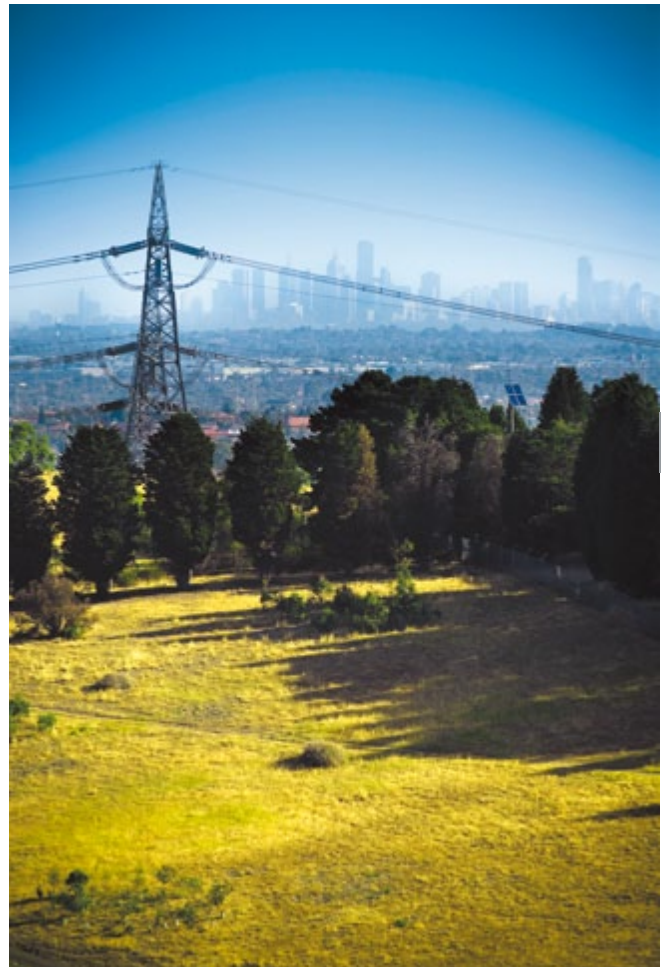
SP AusNet's electricity transmission network delivers power to regional Victoria as well as Melbourne's CBD.
