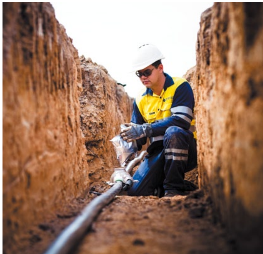
SP AusNet apprentice Alex Gray assists with undergrounding electricity cables in a new housing development.
