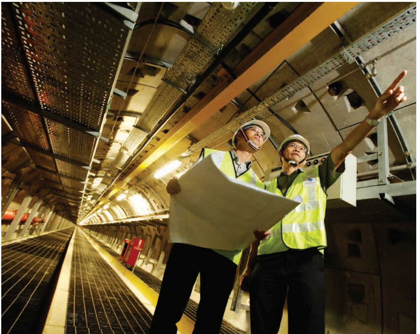
SP PowerGrid's expertise spans the planning and design of Singapore's fully underground grid and gas networks.
