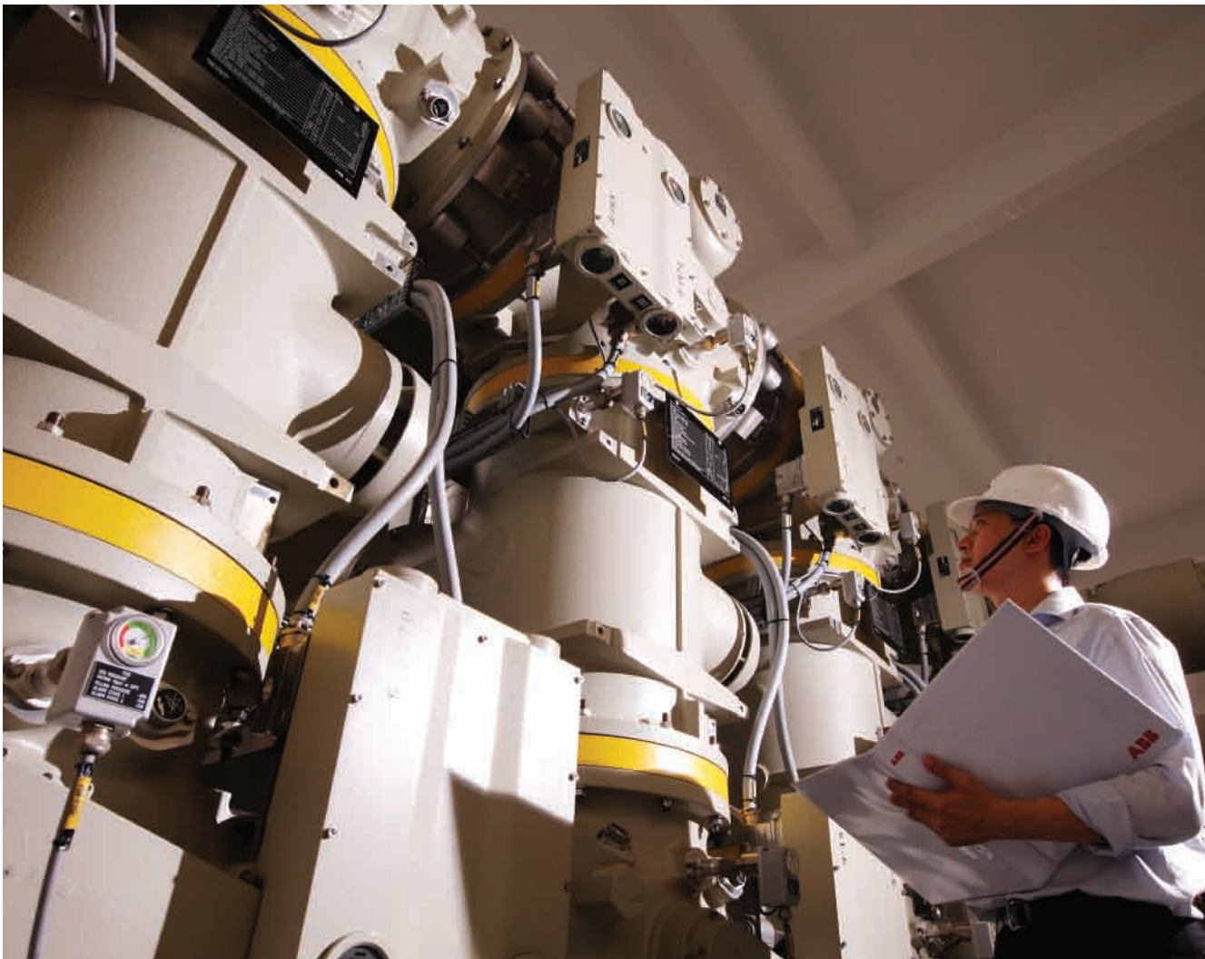
An engineer checking a 66kV switchboard.
