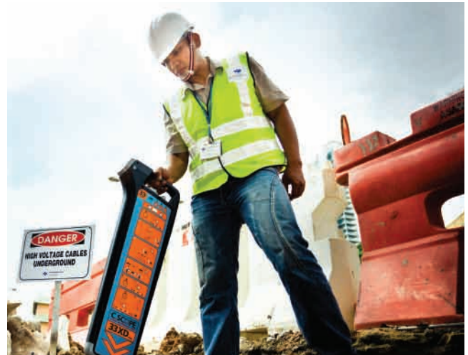
With 29,000km of underground cables to safeguard, SP PowerGrid has to be vigilant where damage prevention of our utility infrastructure is concerned.
