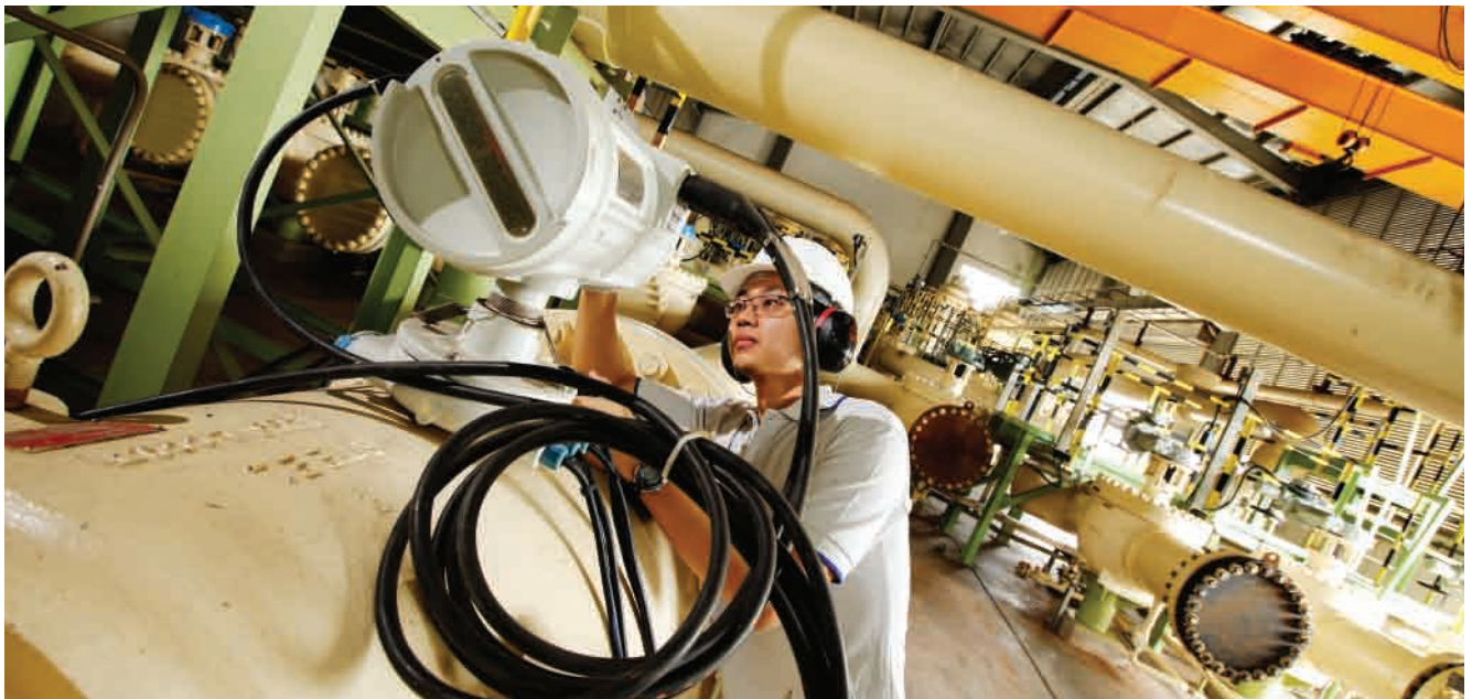
The ultrasonic meter measures natural gas volumes.
