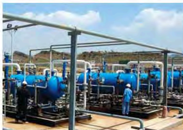
Separators at Nashpa Plant, district Kohat, KPK
