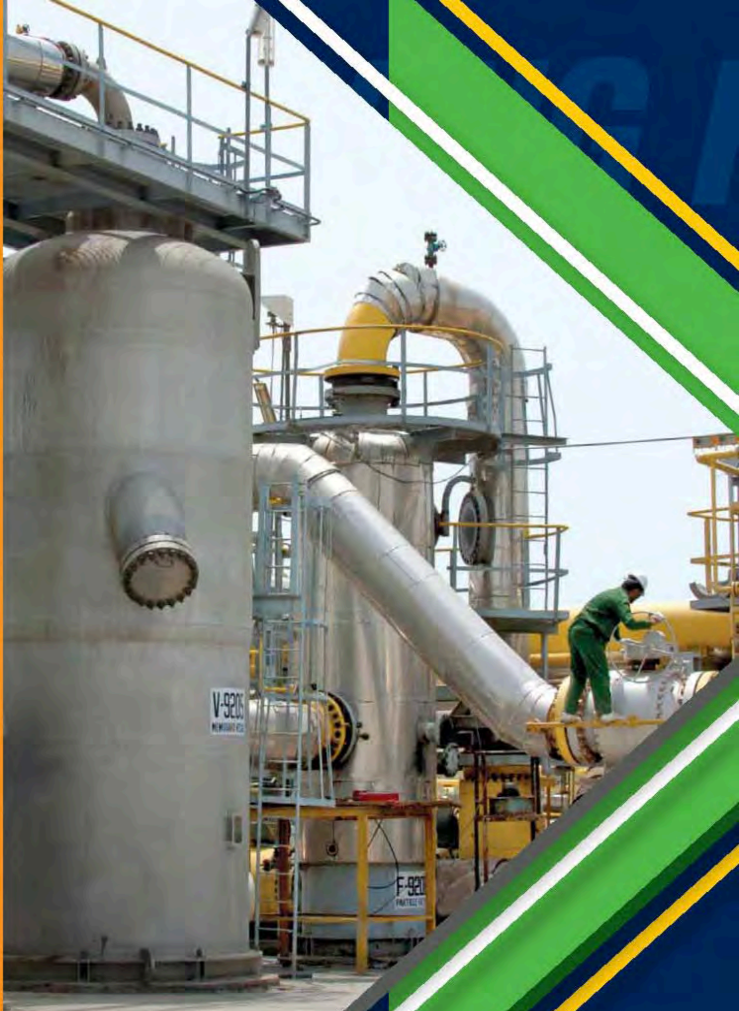
Cedrpur Gas plant, district Ghotki, Sindh.
