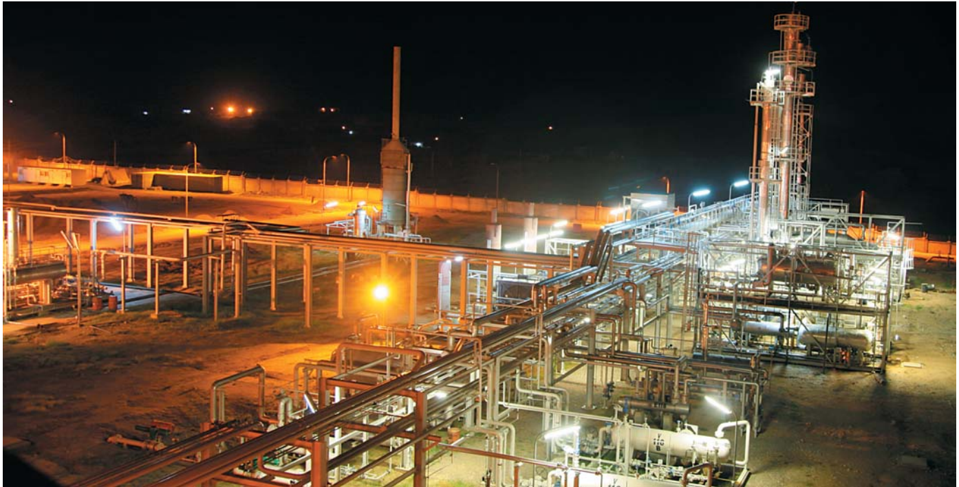
Chanda Gas Processing Plant
