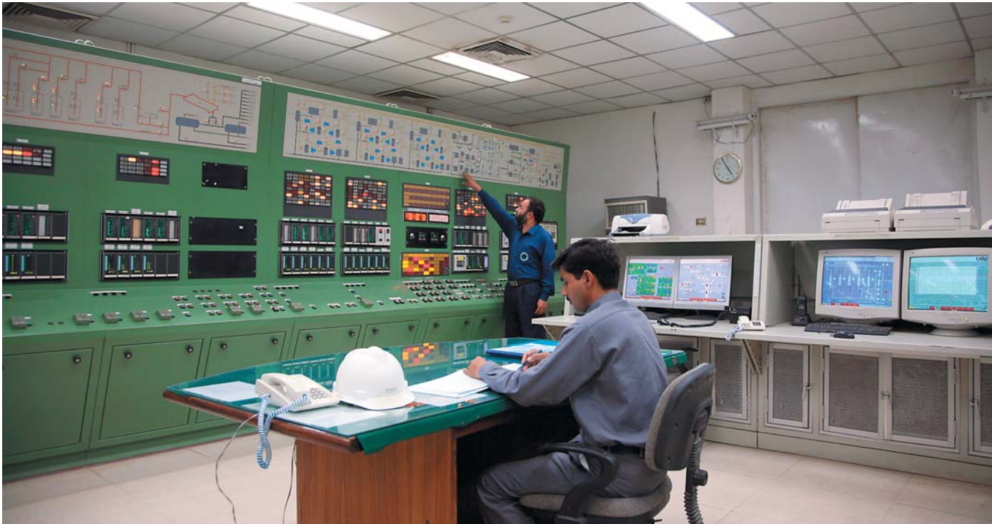
Central Control Room - Qadirpur Gas Processing Plant
