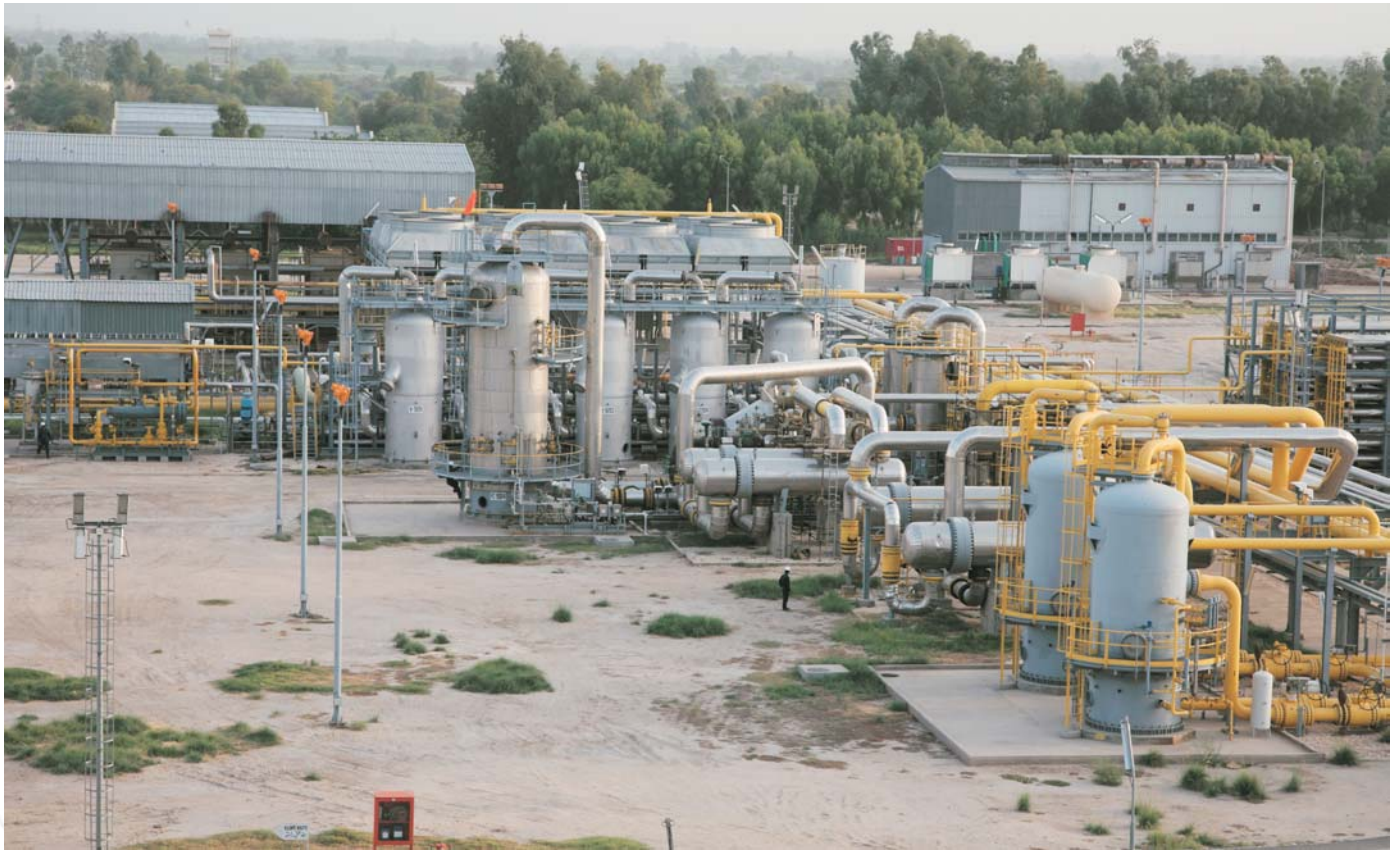
Qadirpur Gas Processing Plant
