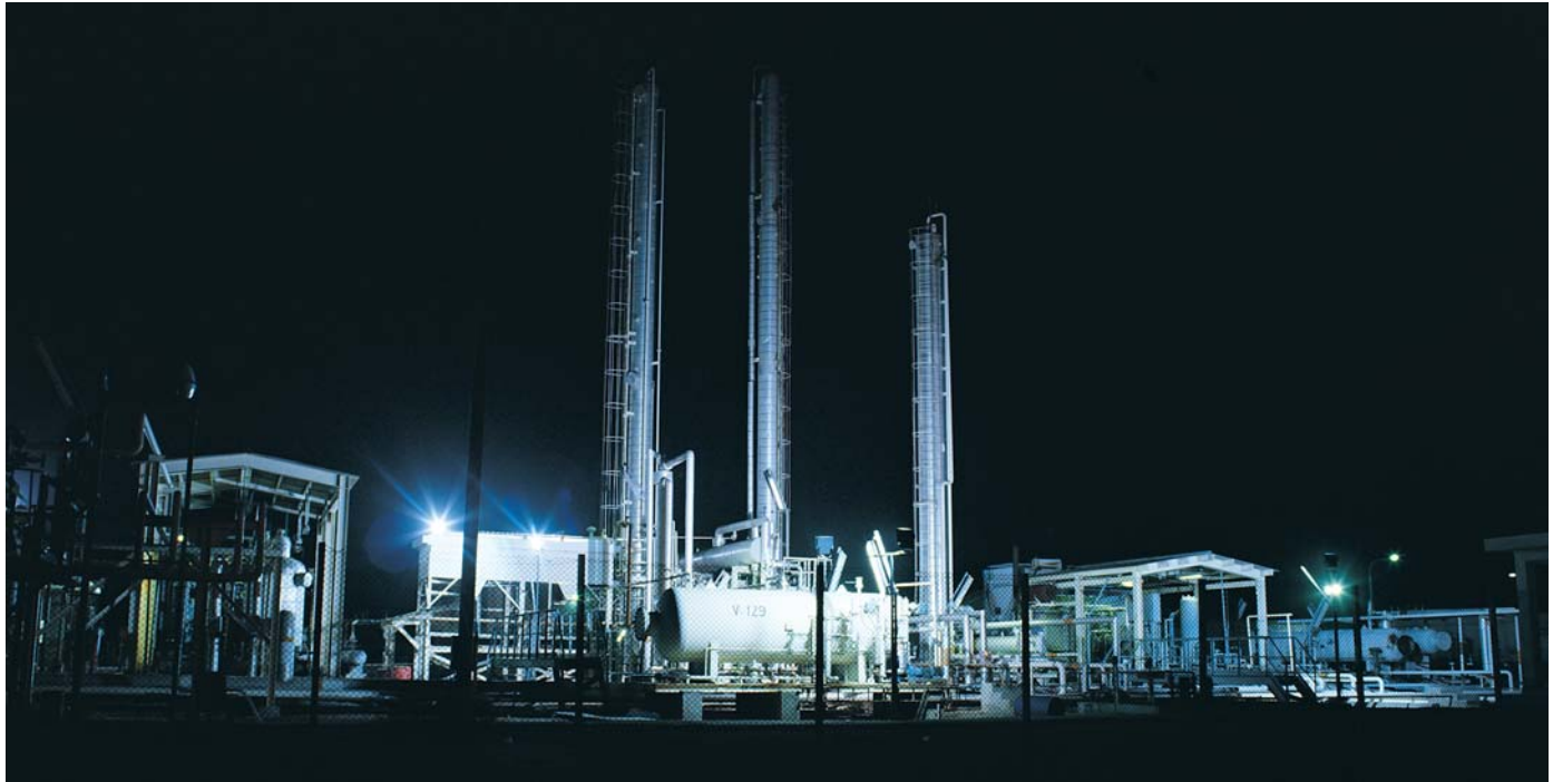
Kunnar LPG Plant
