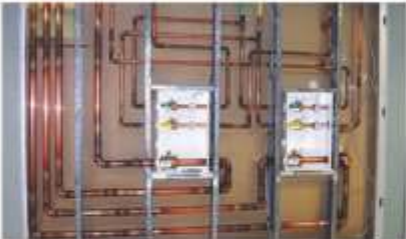
Medical Gas Pipeline
