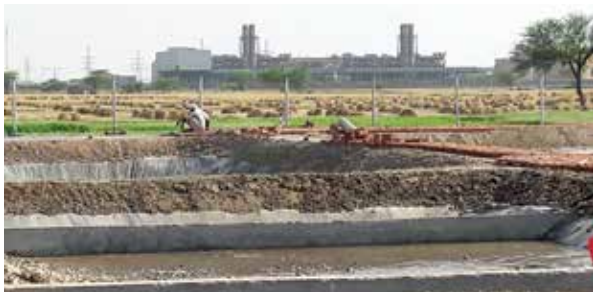
Sewerage Treatment Plant, Poong, Narowal
