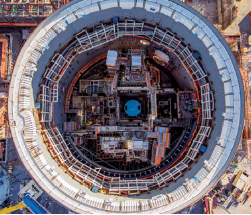
Bird's-eye view of Unit 3 nuclear island under construction at Georgia Power's Plant Vogtle, near Augusta, Georgia
