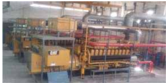
Captive Power Plant
