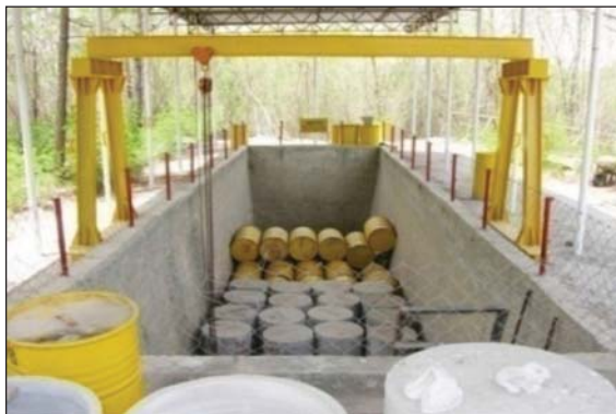
PINSTECH Predisposal Radioactive Waste Management Facility (PPRWMF)
