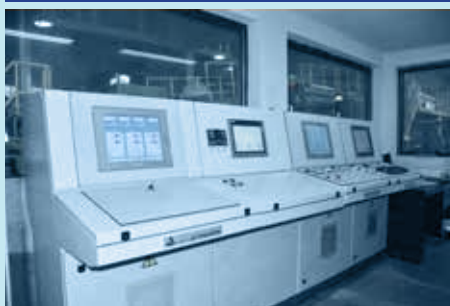
Corrugator Drive Control
