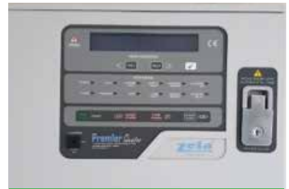
Fire Alarm System
