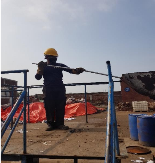
Manual waste feeding in the Incinerator
