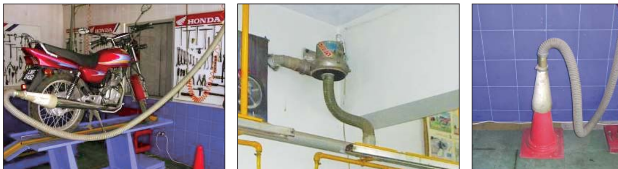
All dealers are required to install Motorcycle Exhaust gases Ducting System in their workshops.
