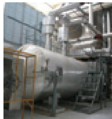
▶ Waste Heat Recovery Equipment
