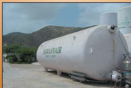
BULK LIQUID STORAGE TANK. (65000M3 CAPACITY)
