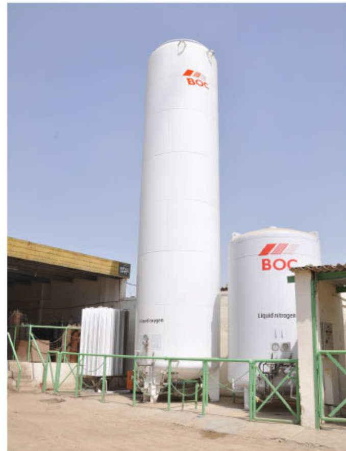
Our largest storage vessel (25K m 3 ) installed at a customer site in Karachi
