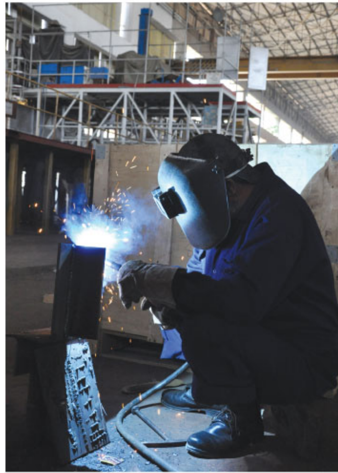
Our gases & equipment being used for fabrication at a large Shipbuilding Complex in Karachi.
