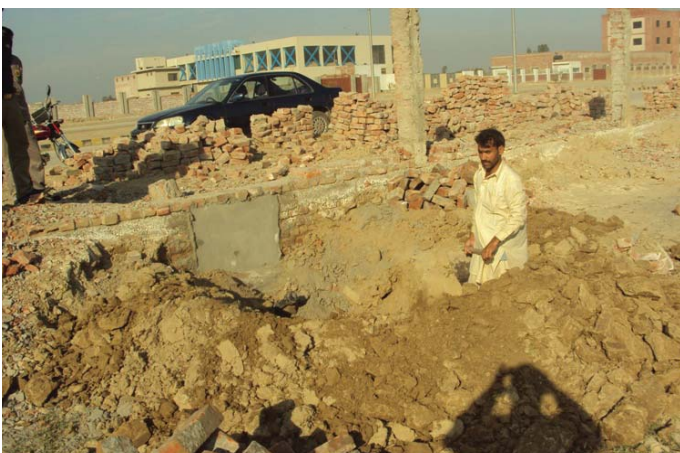
Civil work in progress at Sundar Industrial Estate, Lahore for Company's new state-of-the-art ASU plant
