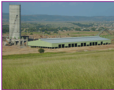
Coal Storage Yard with CF Silo
