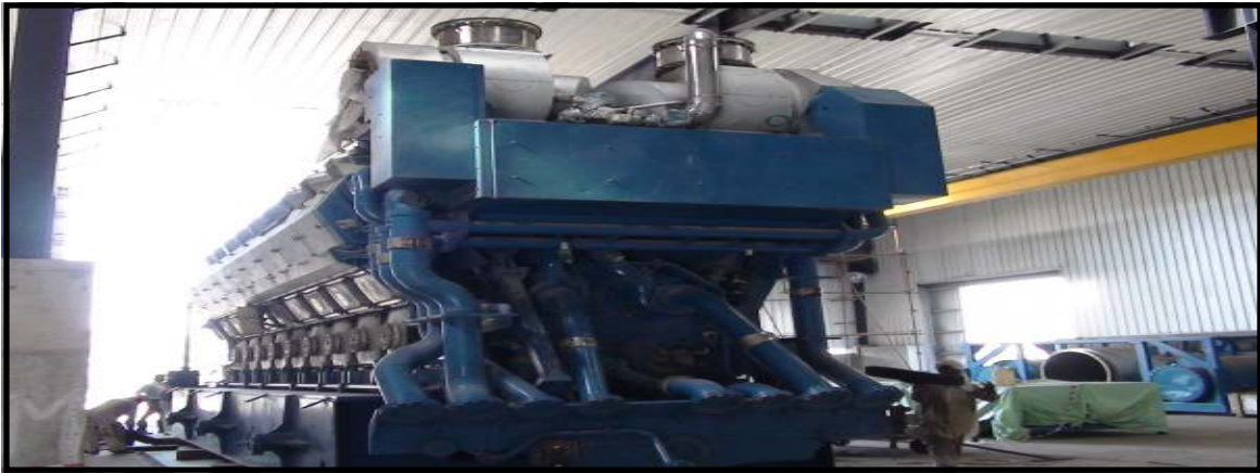
Wartsila Power Plant
